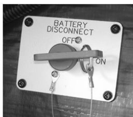
Battery Disconnect Switches
